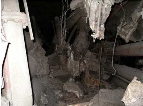
Explosions during ash handling
