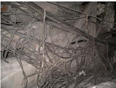
Explosions during ash handling
