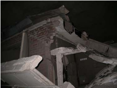
Explosions during ash handling
