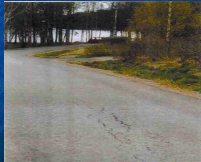
Reference road traditionally renovated Cracks after 1 year
